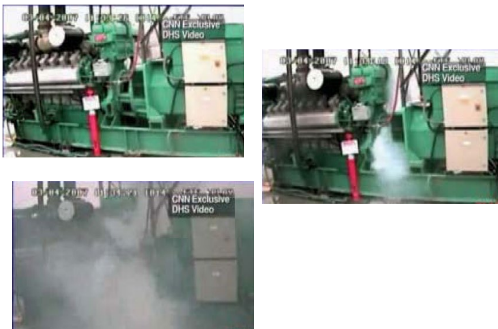
Figure 2 - Aurora Generator Test, Idaho National Lab, INL
